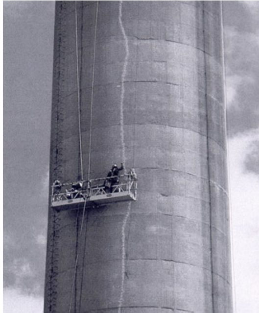
Fig. 2. Exterior repairs normally do not require interruptions in plant process and, despite the heights involved, are simpler to perform than interior repairs. Here, maintenance personnel pressure inject epoxy into a structural crack.
