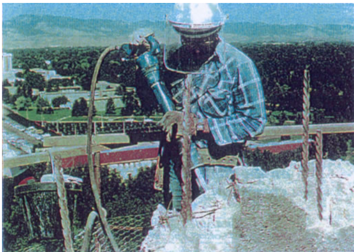
Surface preparation or partial removal is often needed before a chimney is extended. Any height extension affects the stress conditions on the structure by increasing the moments caused by wind and seismic loads on the extension.
